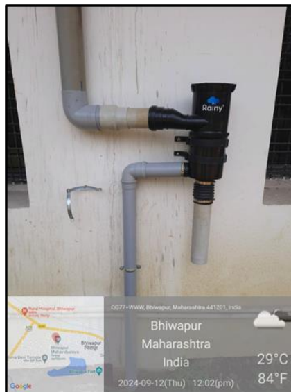
Rainwater harvesting system observed in the campus
