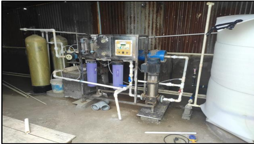
RO Water Units were observed in the Campus
