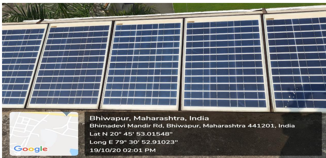
Figure 2.3 :- Solar Plant 4 KWp and Inverter System
