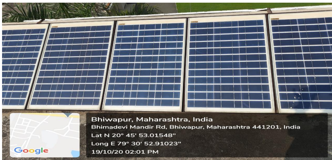
Figure 3.1 : - Solar Plant KWp and Inverter System
