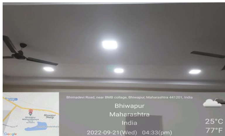
Figure 2.4 :- Electrical Equipment in College
