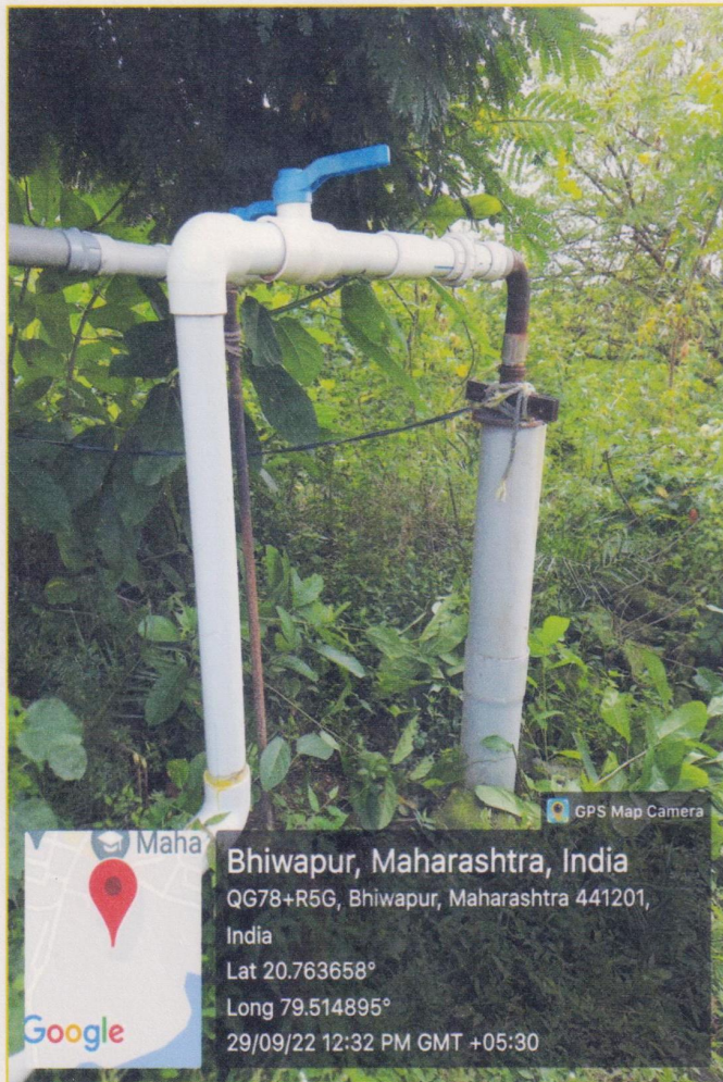
Bore well Near the Swimming Pool
