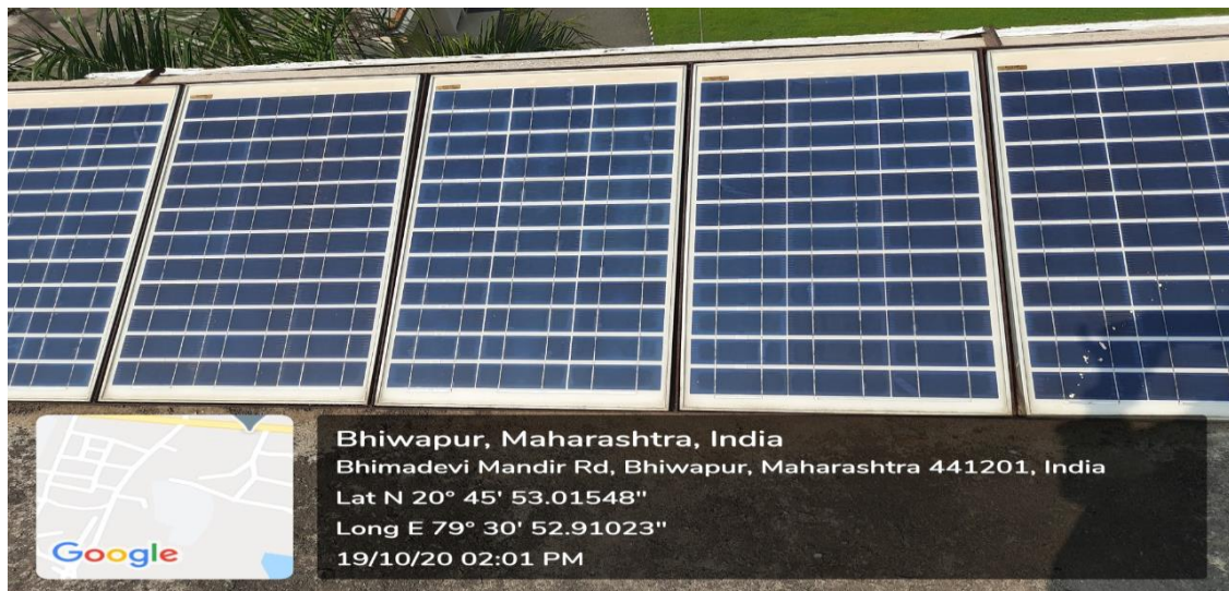
Figure 3.1 : - Solar Plant KWp and Inverter System
