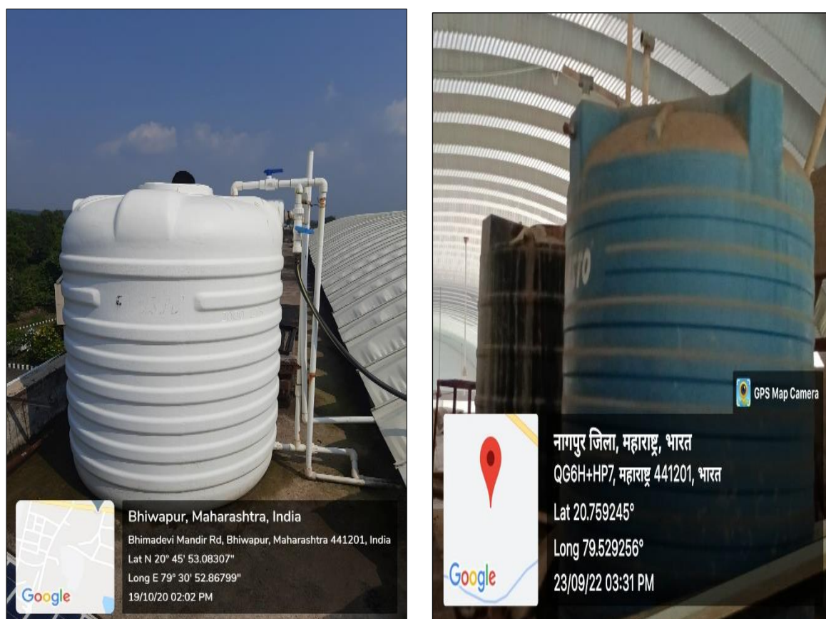
Figure 2.2 :- Water Storage Tank and capacity of College Campus
