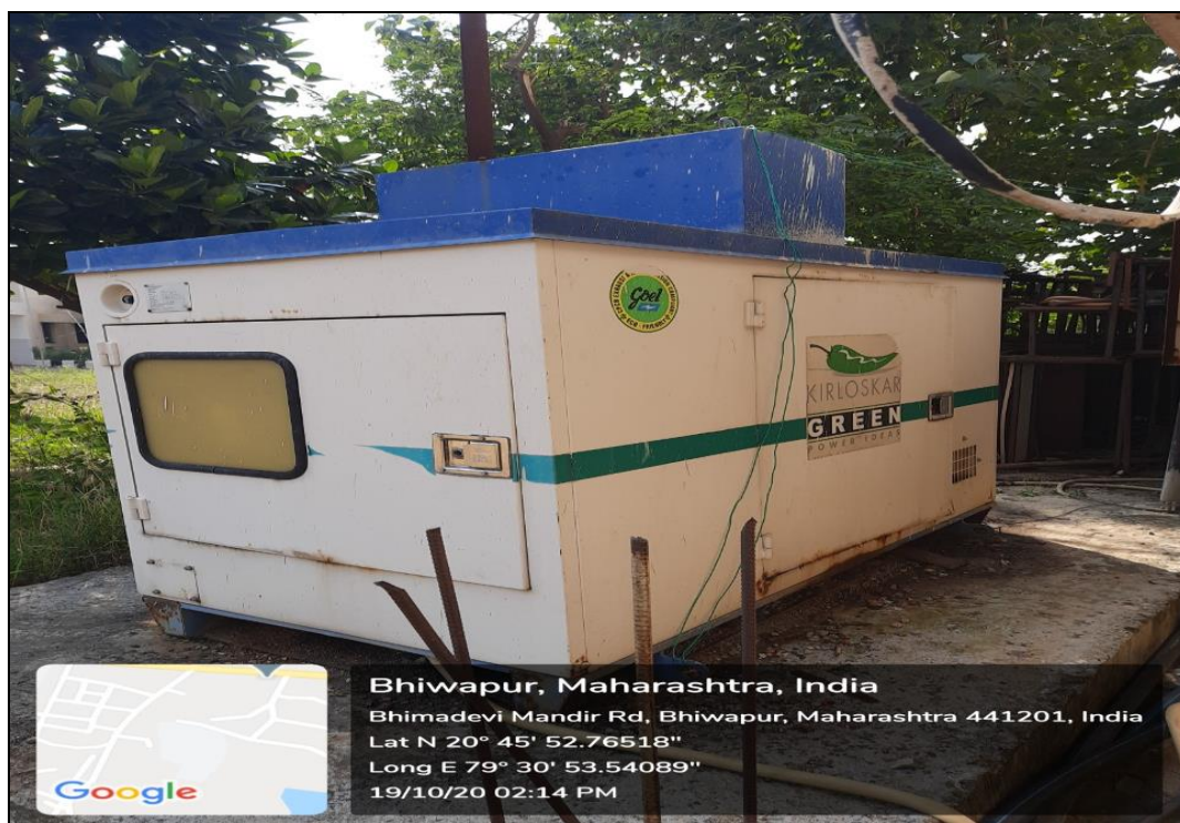
Figure 2.2 :- DG set in Power House
