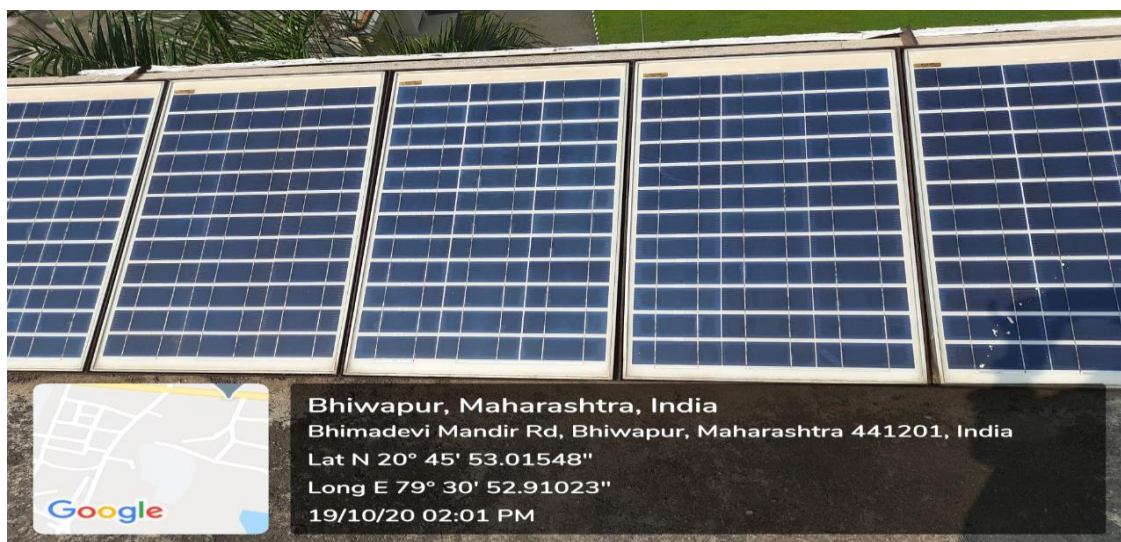
Figure 2.3 :- Solar Plant 4 KWp and Inverter System
